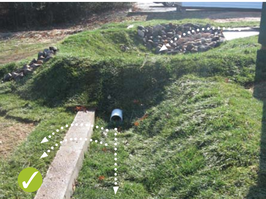
Concentrated flows are collected in small forebay and discharged into 6 inch deep "swale" before overflowing concrete lip as sheet flow (Source: NC State University).
