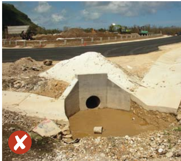
Failure to provide any form of inlet protection. Silt and debris from construction site is conveyed to entrance of inlet from road and unstabilized areas and is then directly discharged.
