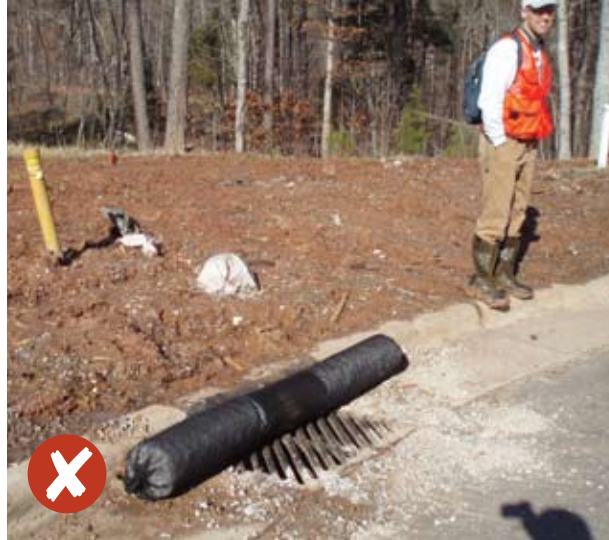
This prefabricated product is not suited for this type of inlet structure. Good extension of device on either side of inlet, however "dirty" flows enter drain directly through grated opening. Consider covering with wire mesh/fabric and/or rock.
