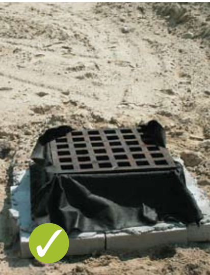
Fabric liner inserted behind grate. Because tearing is common, this practice will require daily inspection and repair.
