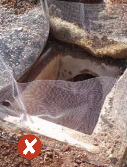
Poor installation and maintenance of wire mesh. Rock missing on two sides of inlet. Use fabric with wire to help filter sediment.
