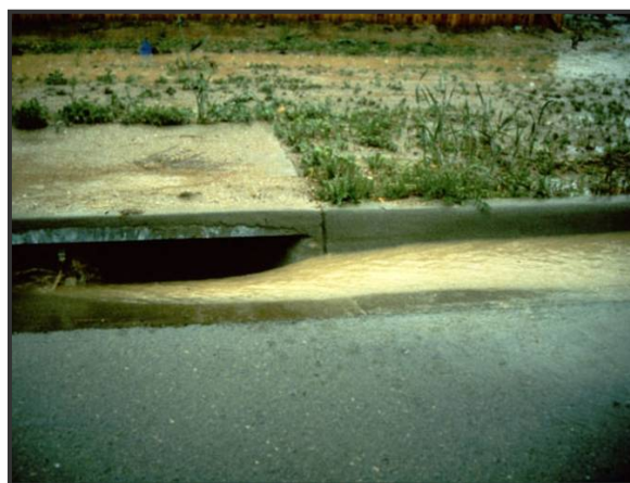
Figure 1.8 Sediment washed into a catch basin during a storm event.
